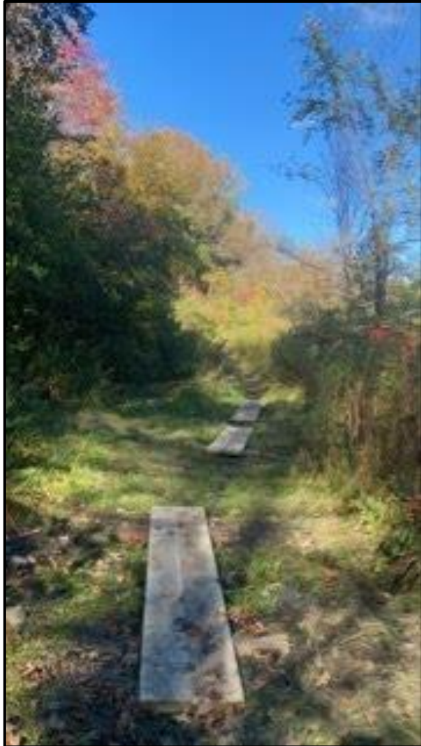
ABOVE: SEVERAL OF THE NEW PUNCHEON INSTALLED TO CROSS OVER A MUDDY SECTION OF TRAIL
