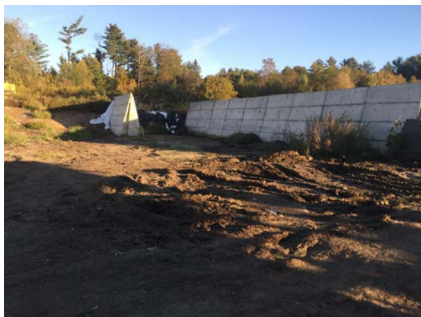
Figure B25. Unstable area at Neddo Farm.
