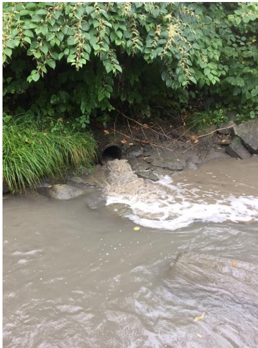
Direct roadside storm water discharge from Boynton St in Barre City
